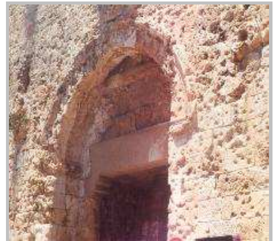
The Zion Gate still shows signs of damage from the battle for control of Jerusalem in 1948.
